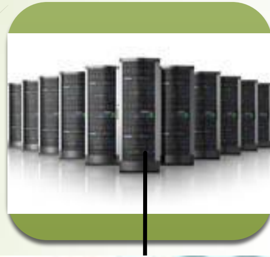
NIDA Datacenter AFIS System
